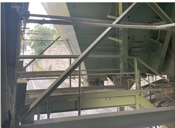
The long narrowing slope of the discharge chute would quickly build up and clog.
