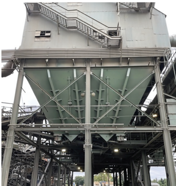
The Tilcon silo/hopper loads both trains and trucks in this dual-lane feeding system.
