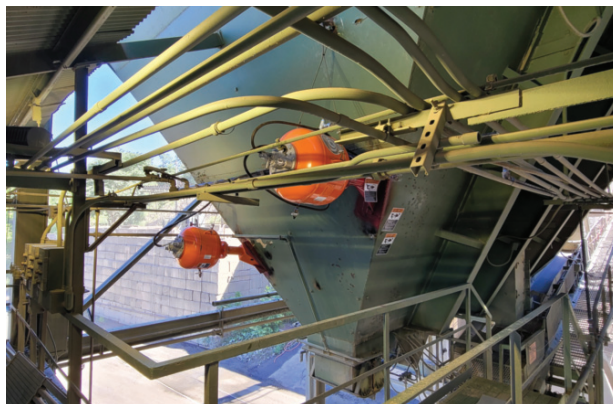
Air cannons are placed in choke points, often indicated by hammer scars from previous attempts to loosen material.
