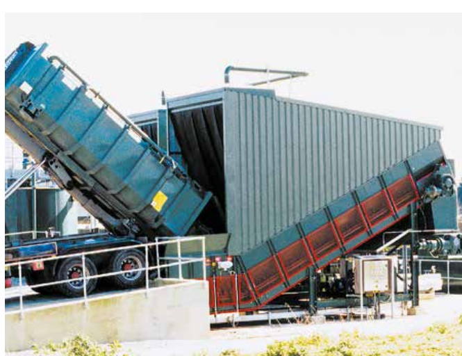
Sludge intake facility with twin screw-conveyor onward transport
