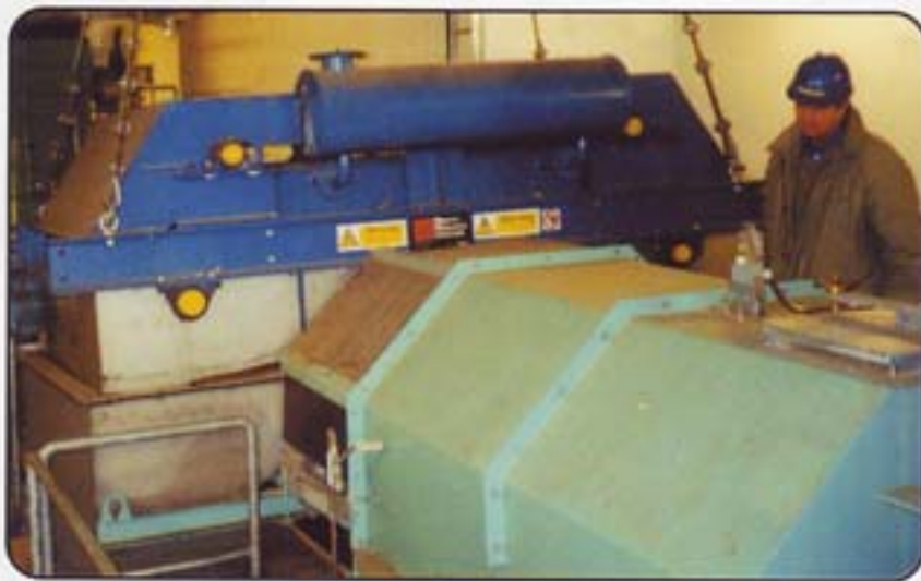
Guarded In-line Heavy Duty Electro Magnet in operation
